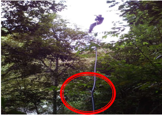
Figure8. Destroyed ordinary aerial cable
