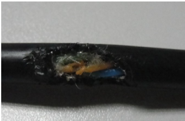
Figure9. Destroyed ordinary aerial cable
